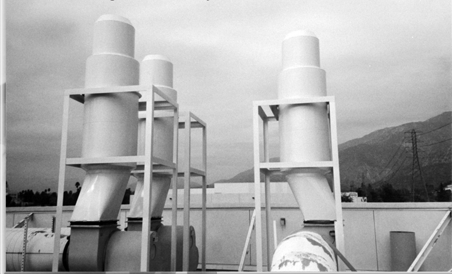
Silencers mitigate community blower noise.
